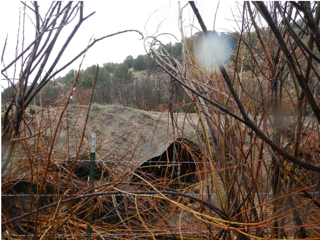
Picture 3 – Inlet damage
